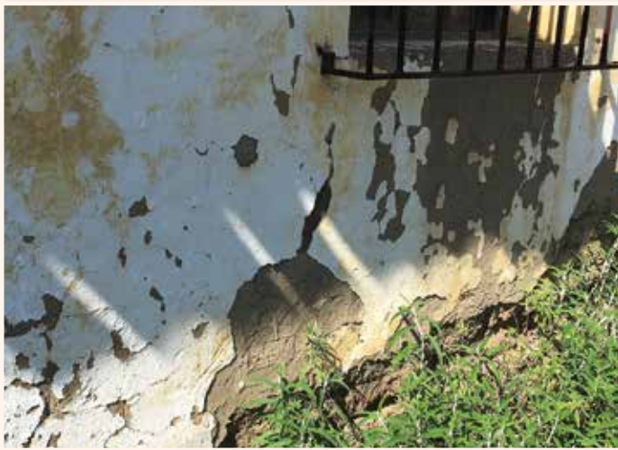
Deteriorated Convento Museum wall
