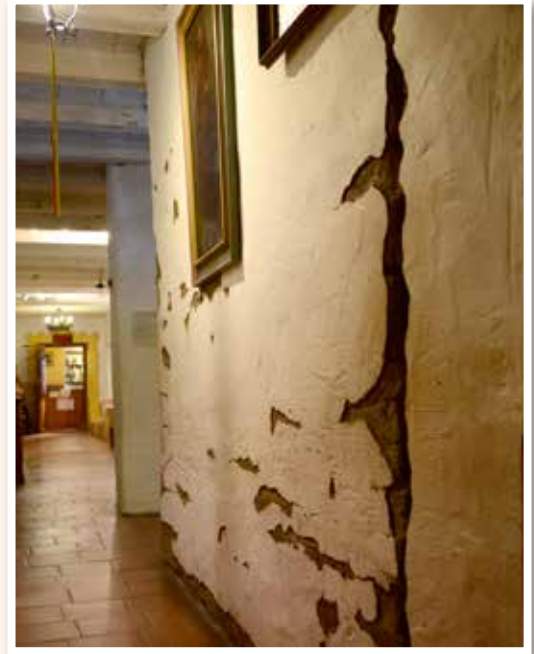
Adobe wall damage inside Convento Museum
