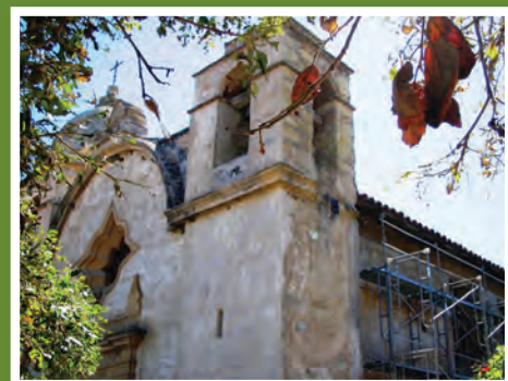
Dome and towers in need of repair
